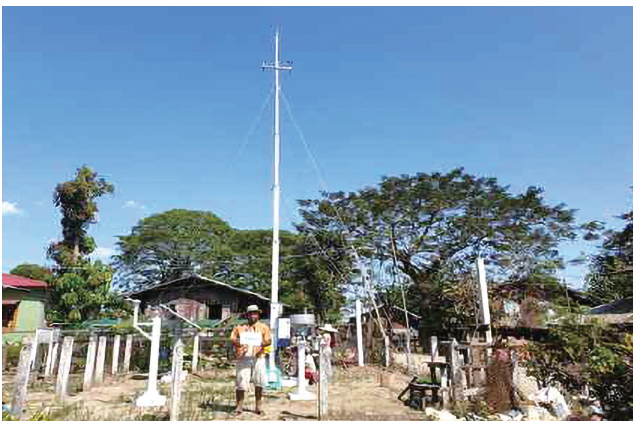
▲ AWS installation site in Homalin
